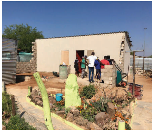
October 2020: First houses built by the community and SDFN at Freedom Square in Gobabis have been constructed.
